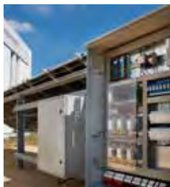
Pv Solar Test Lab
